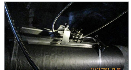
Temporary compressed air flow measuring point with the ultrasonic transducers clamped in Variofix P mounting onto the outside of the pipe. Important in this application: The use of damping mats, minimising signal noise.
