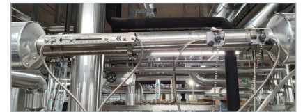
The calibration is carried out by comparing the measured values of the flow meter permanently installed in the skid with those of the test device temporarily attached in series.
